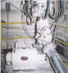
In 12 minutes, CENTRI-SIFTER™ screener sifts 4000 lb (1814 kg) of polymer concrete discharged from pneumatic blender, while eliminating previous screen blinding problem.
